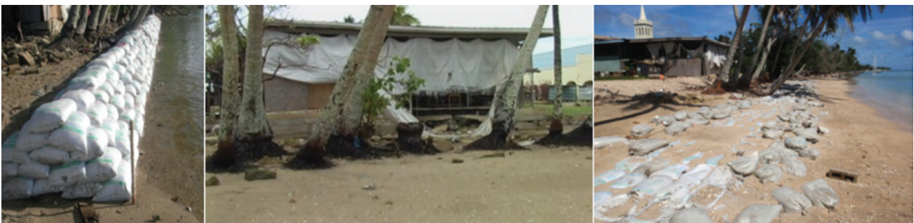
Figure 5: A sea wall project in Hihifo before, during and after Tropical Cyclone Rene (2010)
